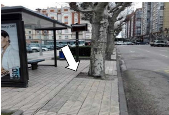
Fig 13. Tree pits not flush with the pavement.
