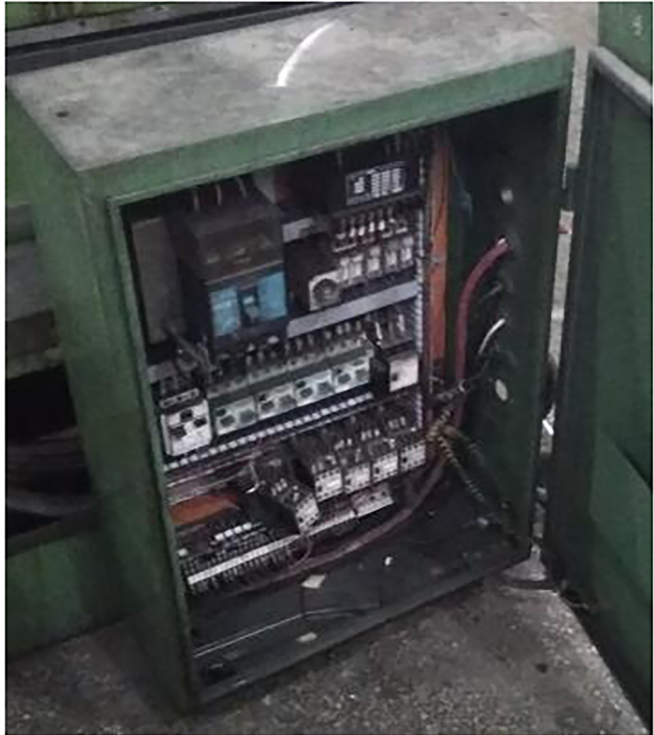
Fig 12. Grinder intensive power control box before reconditioning.
