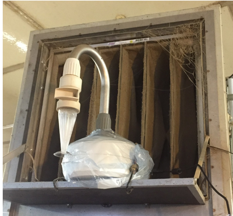
Fig 4. Position of the Coriolis ® \mu Air Sampler in front of the UVC module. The picture shows the Coriolis ® \mu Air Sampler operating on a mounted board in front of the pocket filter for measurements in close proximity to the UVC module.
