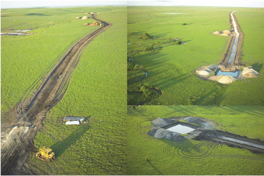
Figure 1. Road and turbine pads for a 150-MW facility in the Flint Hills of eastern Kansas. Over 30 km of new roads and 99 turbine pads were constructed in tallgrass prairie for this project. doi:10.1371/journal.pone.0026698.g001
