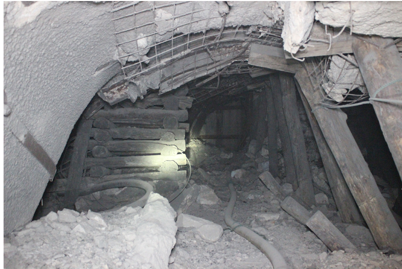
Fig 1. Damage of commonly used steel arch in underground engineering on the field.
